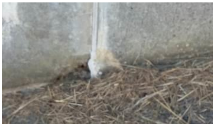
Erosion bajoyer 2 e joint aval passerelle RD
